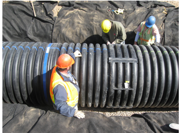
ADS constructed its standard watertight (WT) inline bell spigot joint, and its standard fabric wrapped split coupler connection for each pipe. The connections in each pipe were placed just outside the centerline of the rails. Pipe installation followed standards outlined in ASTM D2321 and in the study.
